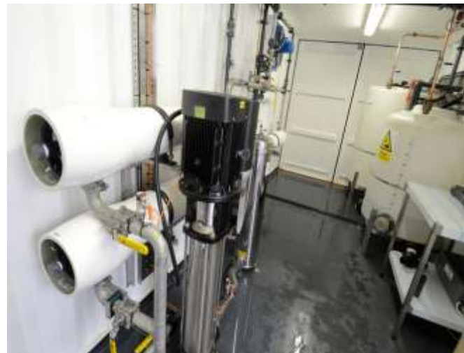
Figure 4: Pilot plant and CIP system
