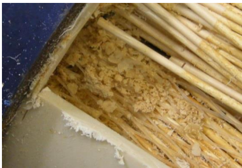
Scaling on UF support surface
