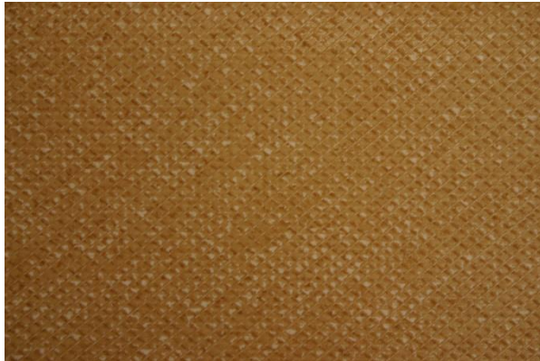
Photograph 21.- General view of membrane surface with significant presence aluminium
