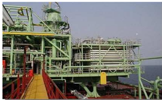
Figure 5: Offshore SR90 membrane plant.
