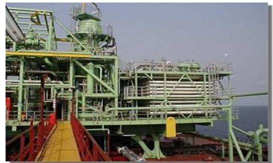
Figure 5: Offshore SR90 membrane plant.
